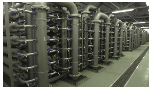
BOTTOM: The Keldgate Ultra Filtration Membrane Plant.
