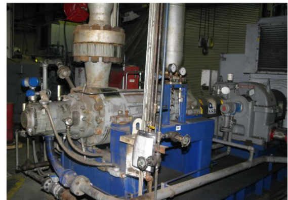
Pump, gearbox, motor assembly
