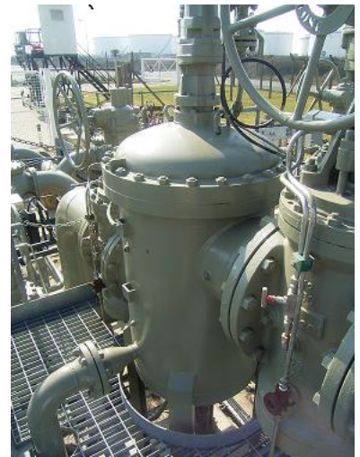
CENTRE & BOTTOM: BOLLFILTER Automatic Filtration System comprising two duty and single standby BOLLFILTER Automatic Type 6.18
