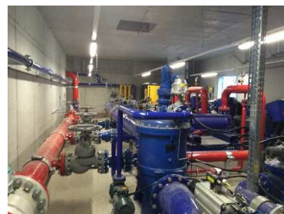
Picture 3: Filter system in the pump station
