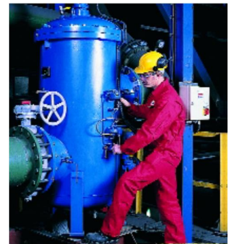
BOLLFILTER Field Engineer, carrying out routine maintenance.
