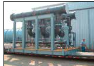
Filtration unit for injection water with three BOLLFILTER Automatic type 618, DN 400
